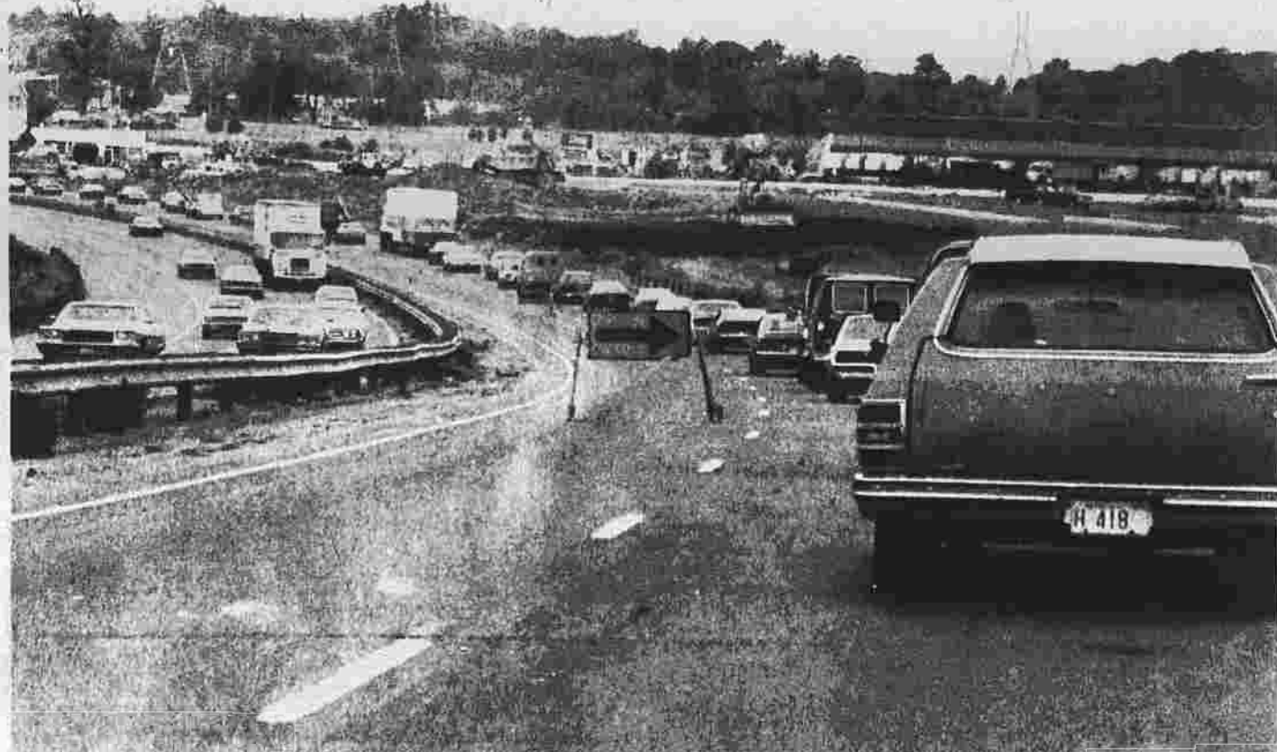
Traffic backs up this morning as it is forced into a single lane on westbound Interstate 86 a couple of miles east of the J.C. Penney warehouse. Interruptions in the highway's traffic flow, required by work on the Tolland Turnpike overpass, are expected to continue until the overpass work is complete. The overpass work is part of the larger I-86 reconstruction project.
